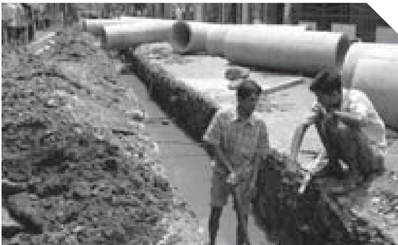
Laying of sewerage line need to consider the ground water flow path
